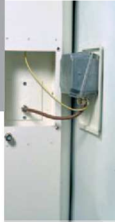
Recessed terminal box / disconnect switch.
